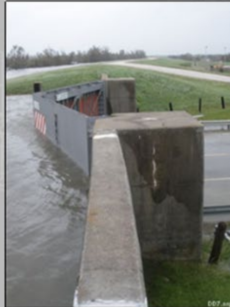
Road closure gate
