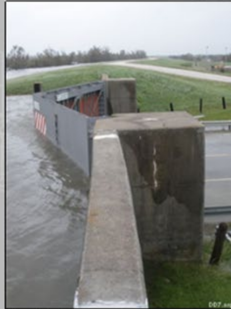
Road closure gate
